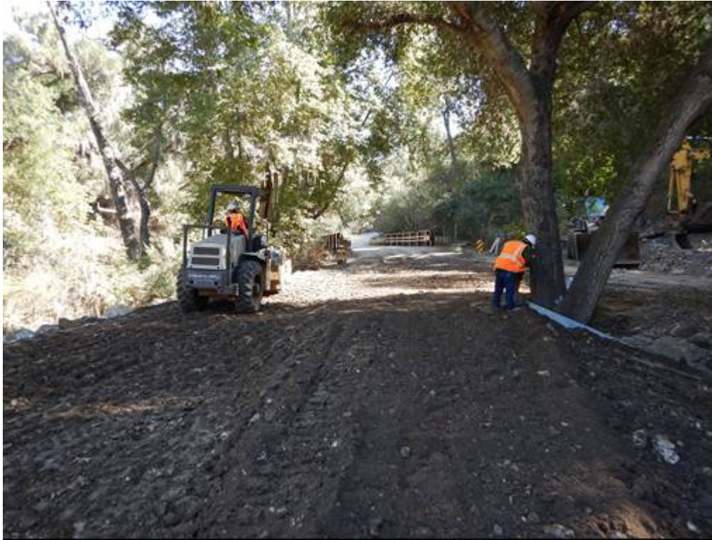
Figure 3: Installing road embankments; metal plate tree well can be seen on the right.
