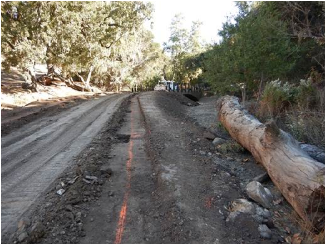
Figure 5: Building the 4 foot wide road berms on the alignment with the guardrails.
