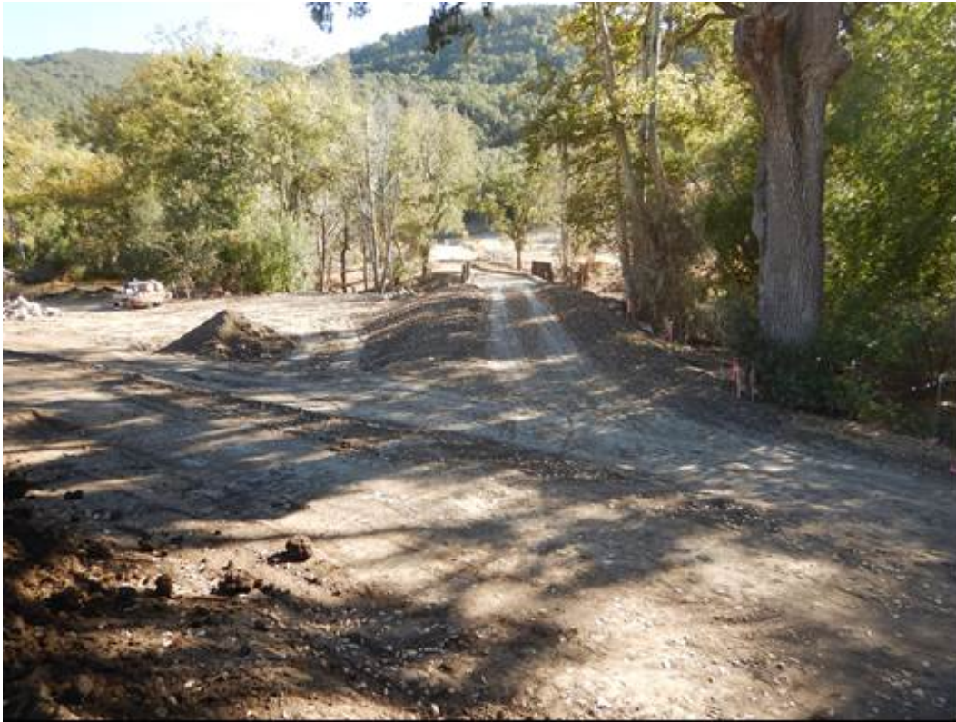
Figure 5: Drainage low point on north side approach road to the bridge.
