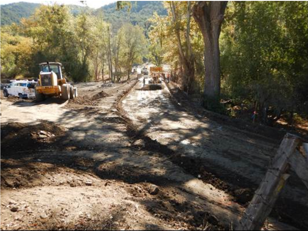
Figure 8: Preparing for road base installation on the north side of the bridge.
