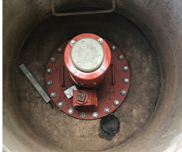
Air Vent 495+30 After
