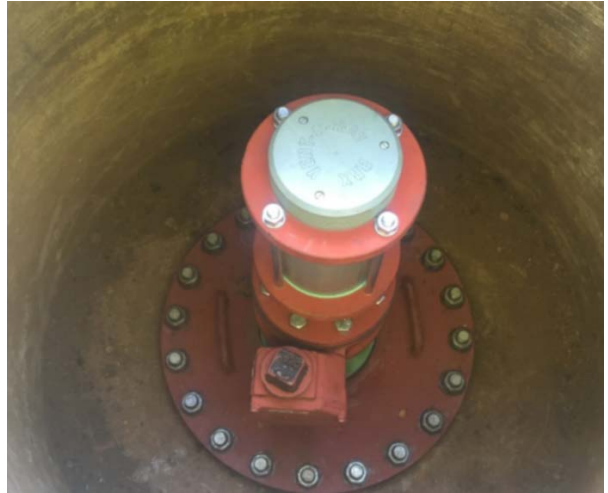
Air Vent 352+07 After
