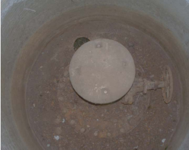
Air Vent 495+30 Before
