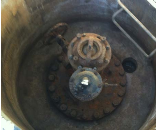
Air Vent 352+07 Before
