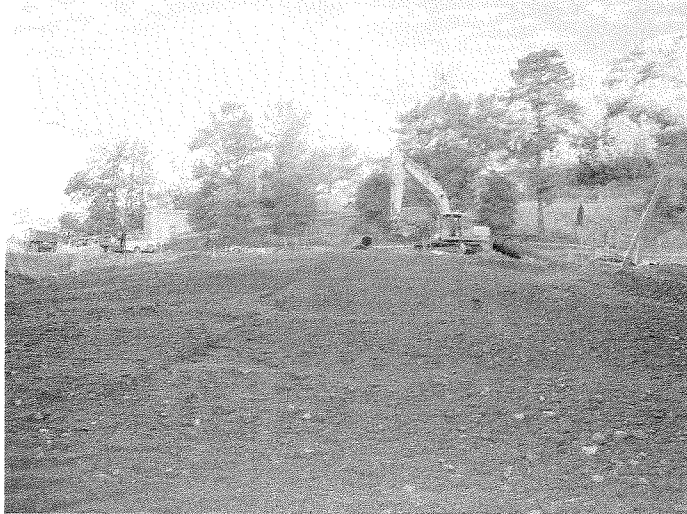
Picture 2 – Debris Dam
