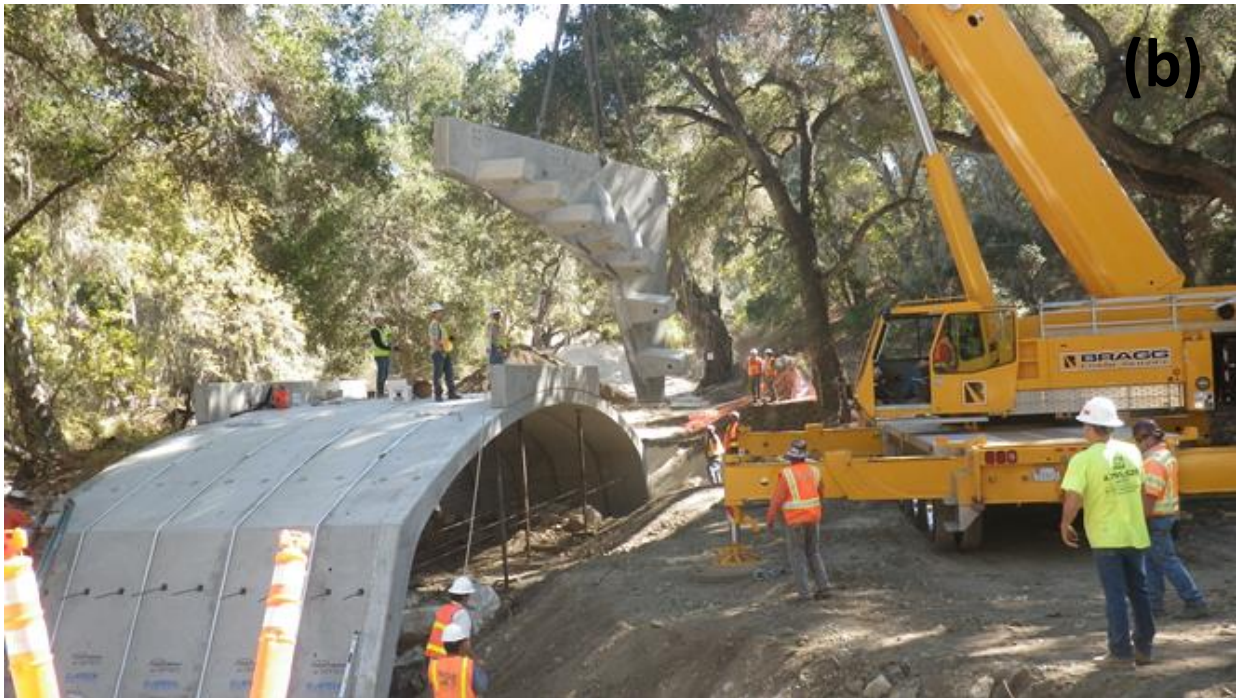
Figure 6: Bridge installation of (a) the first arch and (b) first headwall piece.
