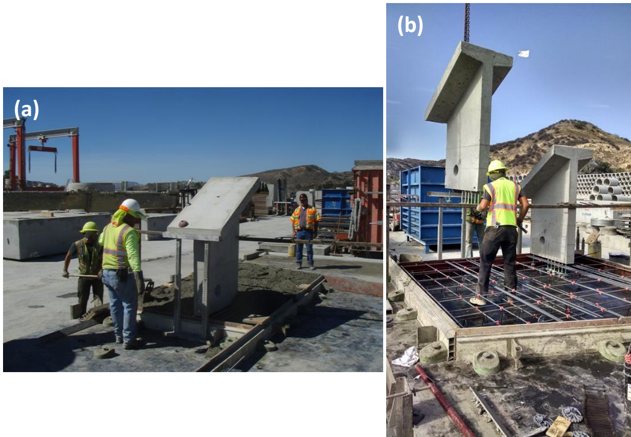
Figure 2: Pre-Con bridge fabrication of a (a) one and (b) two soil anchor wing wall.
