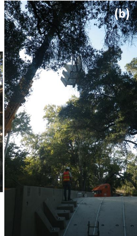
Figure 7: Bridge installation of wing walls on the (a) downstream side and (b) upstream side that had to be lifted over the tree canopy.
