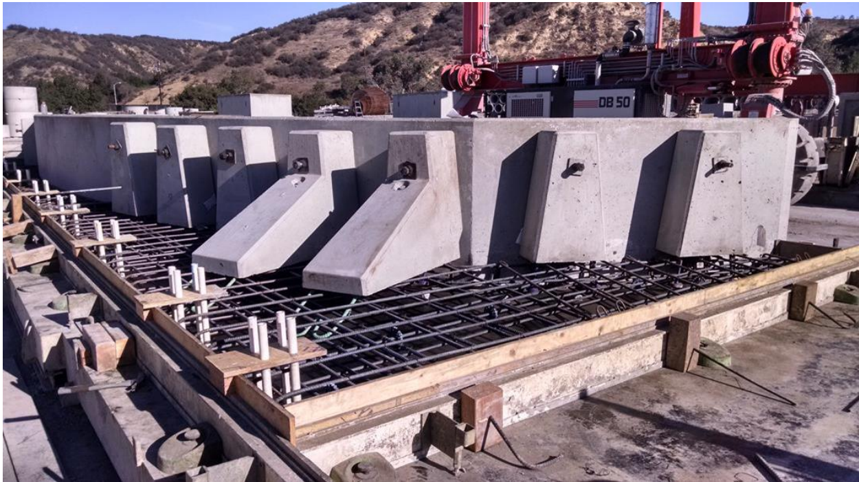
Figure 4: Pre-Con bridge fabrication of the head wall on one of the arches.
