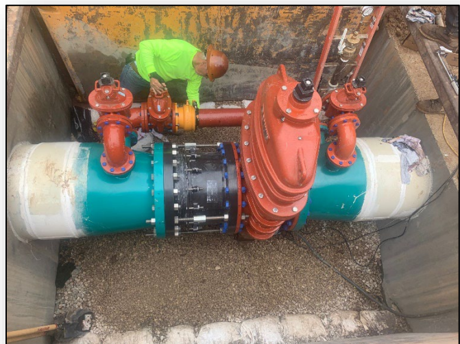
La Mirada Piping and Valve
