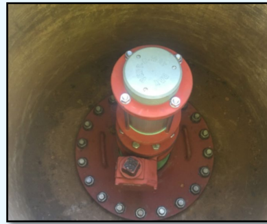
Air Vent 352+07 After
