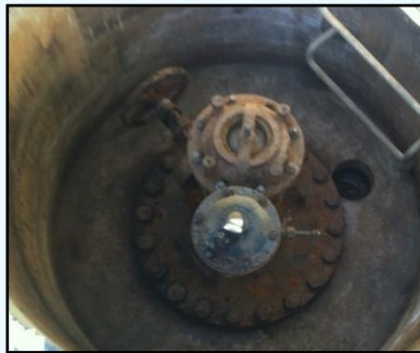
Air Vent 352+07 Before
