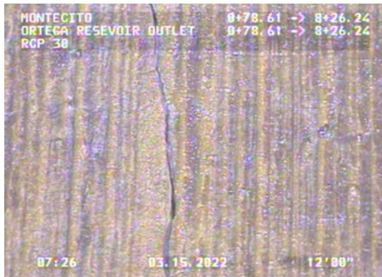
Internal view of crack which caused the leak in the outlet piping outside of the control station in February 2022.
