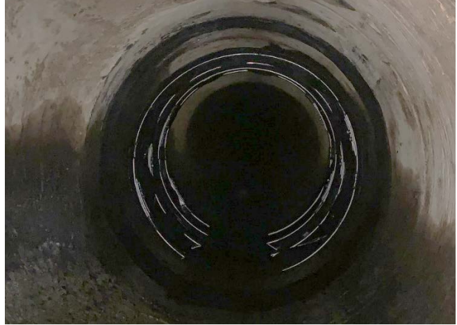
Hydratite seal through the crack area
