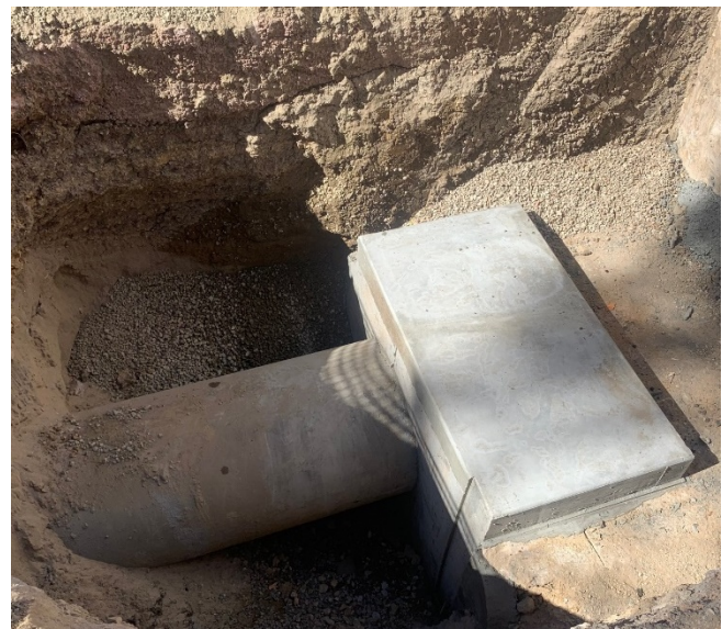
Concrete block supporting pipe and leak (note internal Hydratite seal extends 18 inches beyond edge of concrete block).
