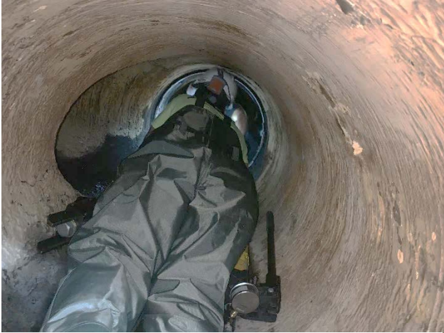
Hydratech technician installing the Hydratite internal seal (EPDM rubber sleeve seal against the pipe wall with stainless steel bands).
