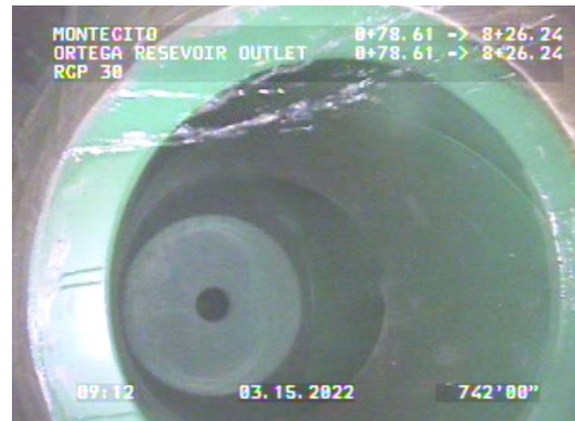
Internal view of the fusion-bonded epoxy coated tee which is located inside the reservoir. Note the small leak where the tee connects to a baseplate that is bolted to the reservoir floor.
