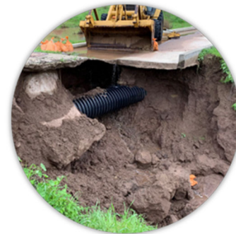
Figure - Lauro Reservoir Bypass Channel Washout January 2023 Winter Storms
