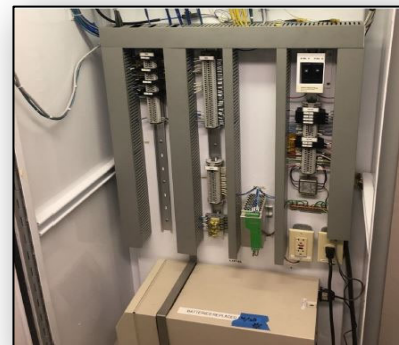
SCADA Control Panel
