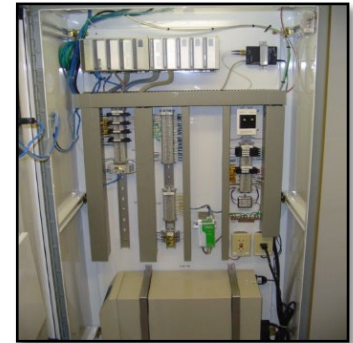
SCADA Control Panel
