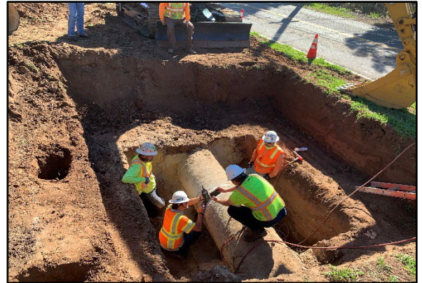
La Mira Isolation Line Valve (Installed 2022)
