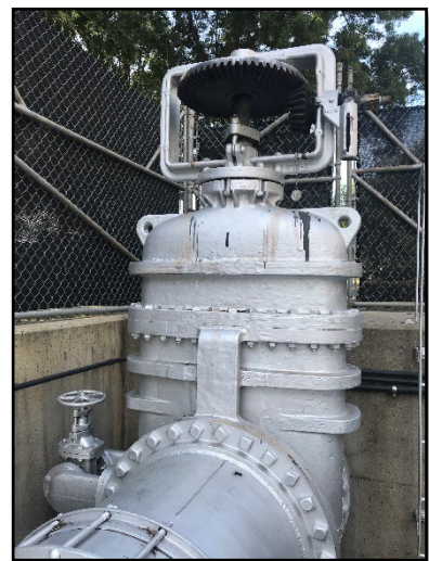
Sheffield Control Station Valve
