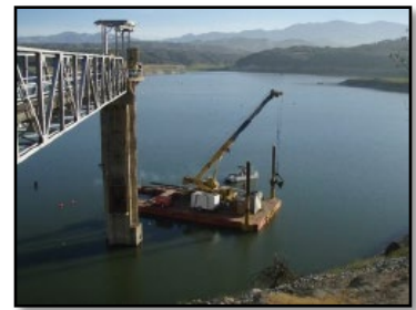
EPF Pumping Facility
