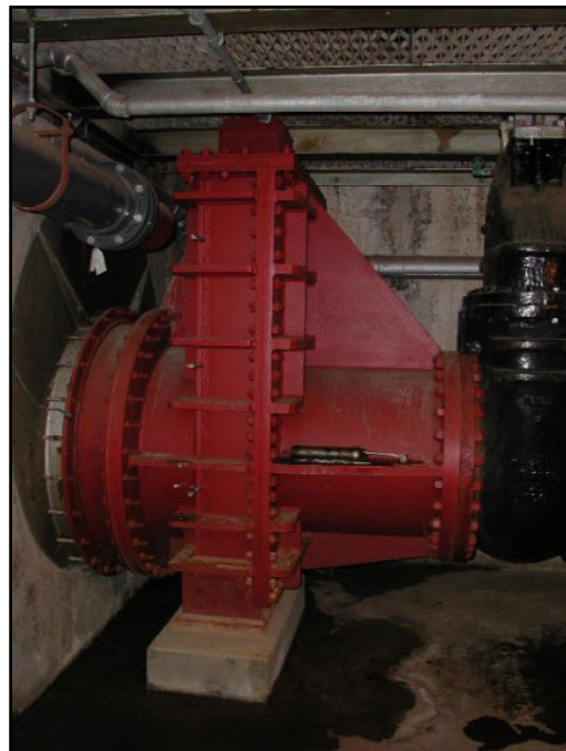
North Portal Jet Flow Control Valve
