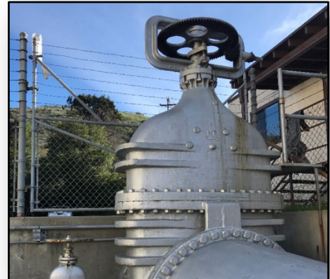
Lauro Control Station Valve
