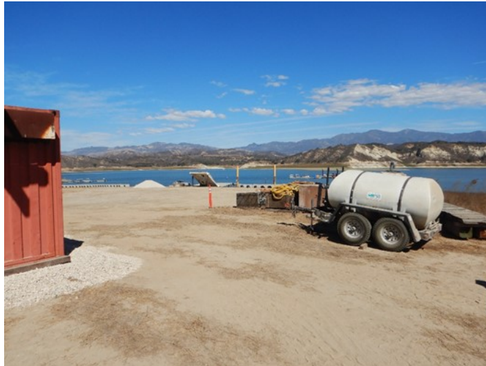
Exhibit 1: The Oak Tree Program water trailer at the staging area for the Secured Pipeline Project for general water supply for the contractor.
