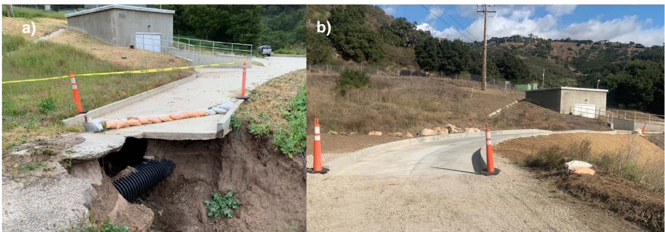
Figure 2. Lauro Reservoir Bypass Channel Road Repair - (a) washout and cantilevered concrete channel and manhole after 2023 storm event; (b) completed repair and concrete channel extension to mitigate for future damages.
