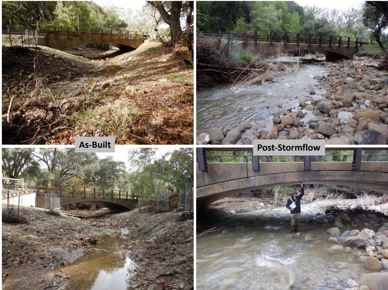
Figure 1: Quiota Creek Crossing 5 As-Built and post-storm condition.
