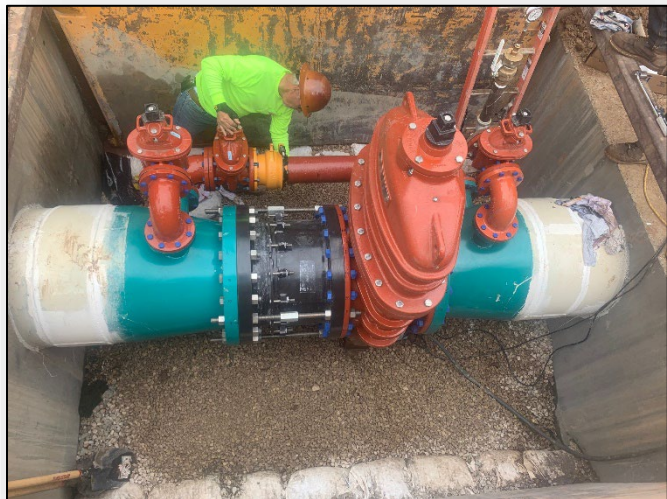
La Mirada Piping and Valve
