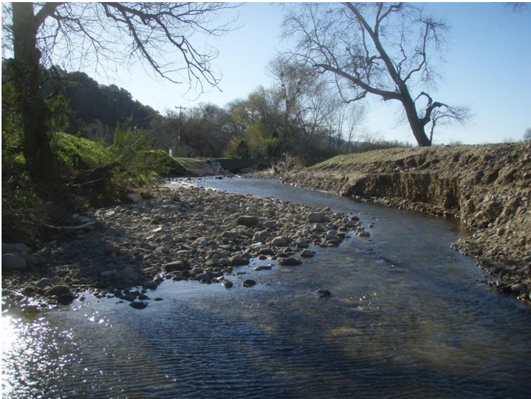
Figure 4: Right and left bank erosion upstream of the culvert (2/28/17).
