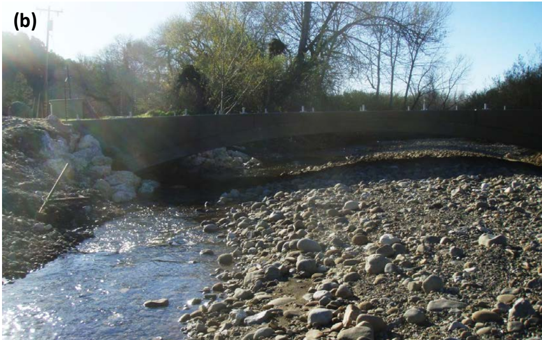
Figure 5: The Quiota Creek Crossing 0A bridge with the (a) As-Built condition in December, 2016 and (b) the current condition in March, 2017 showing the change and specifically the deposited cobble bar.
