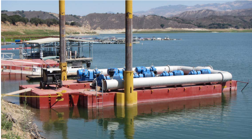
Figure 3. Photo of EPF Pump Station during construction. Not shown is the shipping container that houses the electrical switchgear and variable frequency drives and a wooden platform constructed across the center opening.
