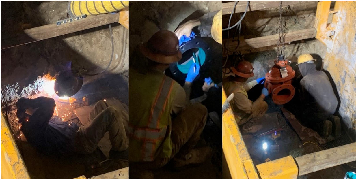
Welding a new flange on the South Coast Conduit and installing a new isolation valve for turnout
