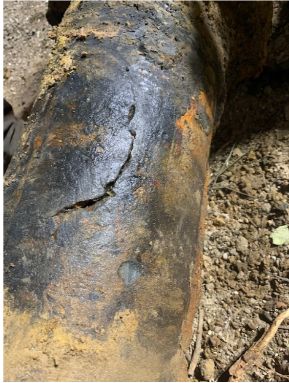
Crack in Original Cast Iron Turnout Piping
