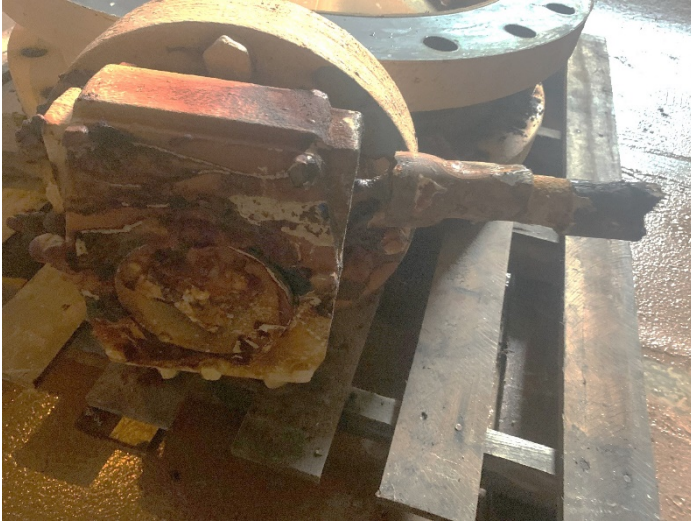
Corroded actuator on existing, inoperable valve
