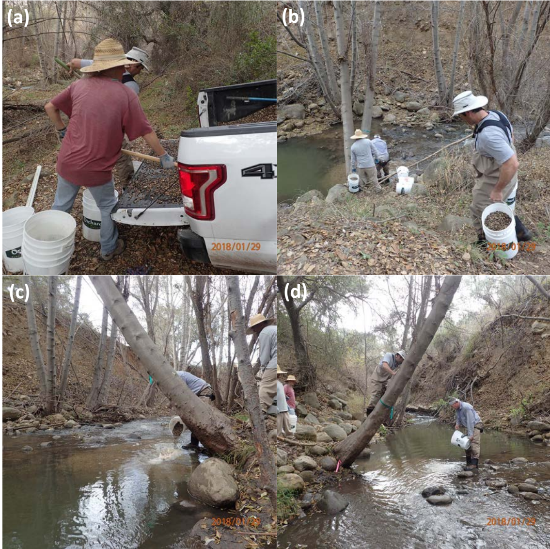
Figure 73: Gravel augmentation in Hilton Creek at the Spawning Pool (a) loading washed gravel into 5-gallon buckets and (b-d) hand placing gravels at the tailout of the habitat.
