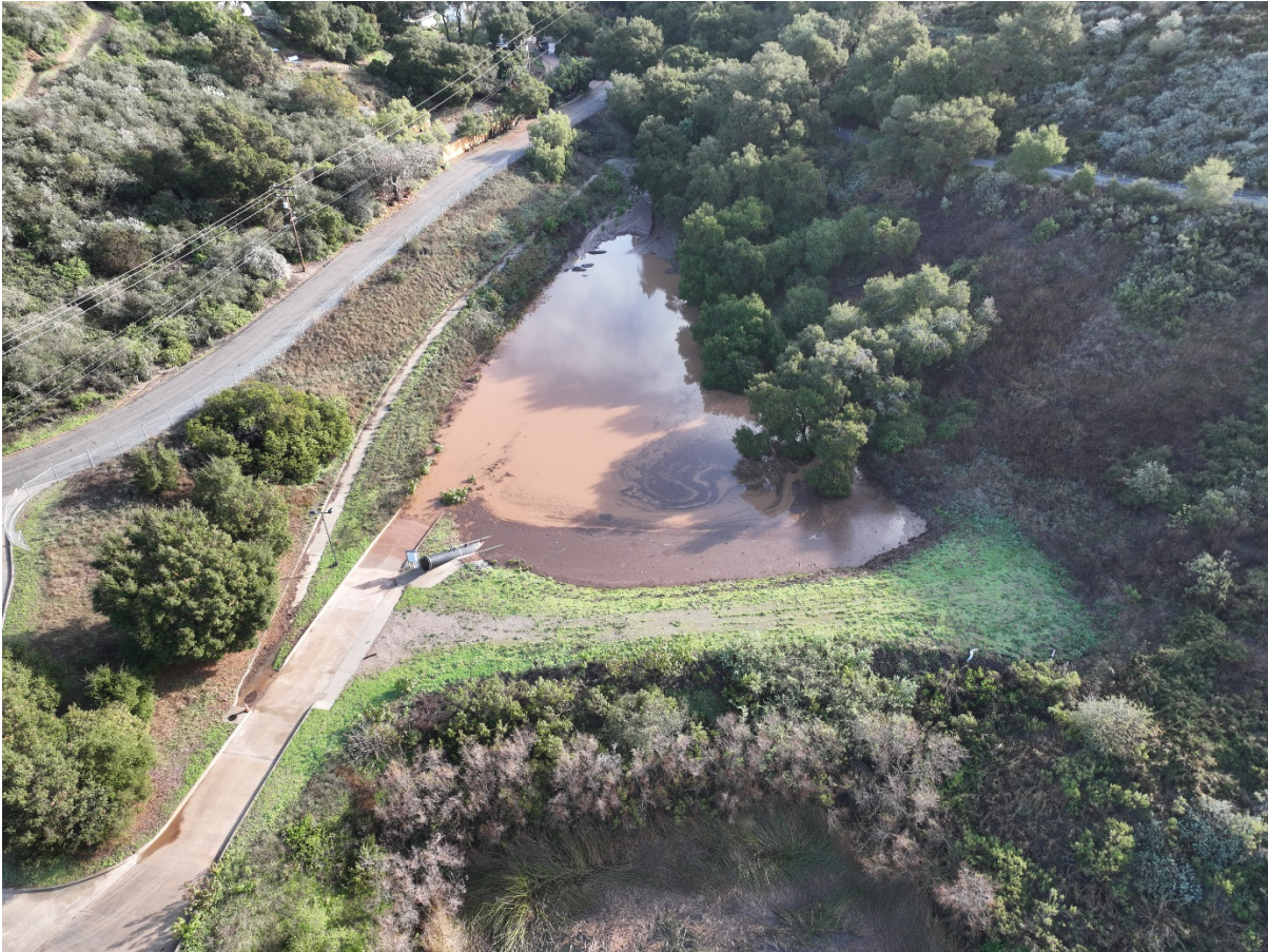
Figure 1. Lauro Debris Basin filled with stormwater and sediment following the January and February 2024 storm events
