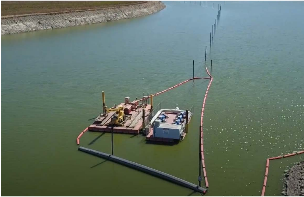
Figure 2. Log booms surrounding Emergency Pumping Facility
