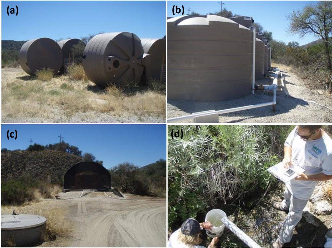
Figure 61: Hilton Creek Water Tanks (5-thousand gallons each): (a) arrival of the tanks, (b) installation, (c) shade protection, and (d) measuring trickle flow at 0.03 cfs.
