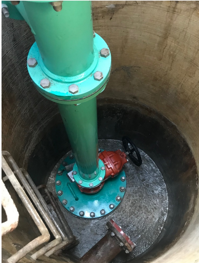
Blowoff Station 552+52 with riser nozzle abandoned, new outlet through blind flange, new valve, and raised discharge pipe.
