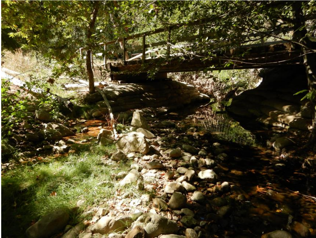
Figure 1: Pre-project condition looking south under the sub-standard temporary bridge with damaged low flow culvert below.
