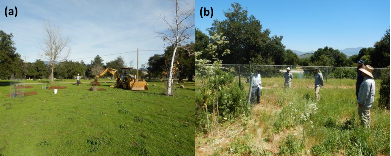
Figure 18: Oak Tree Program showing (a) digging with a backhoe and planting Year 11 trees at Santa Barbara County Park, and (b) hired arborist training staff on Grow-Tube removal and tree tying.
