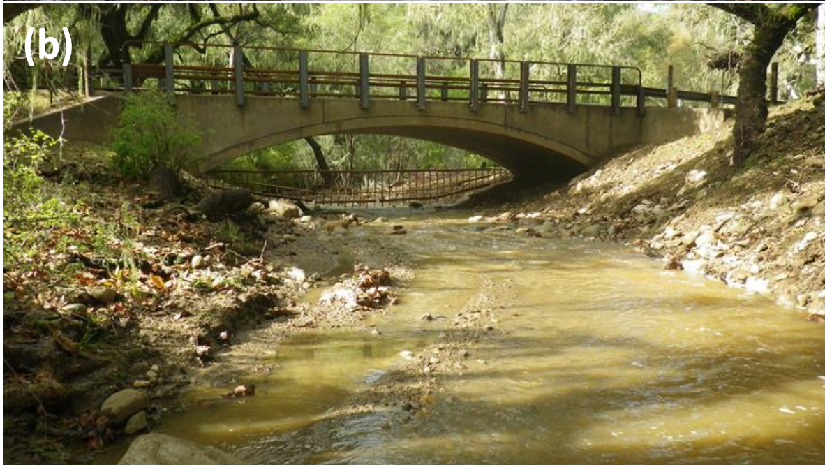
Figure 4: The project with Quiota Creek flowing looking (a) upstream and (b) downstream on 3/6/16.
