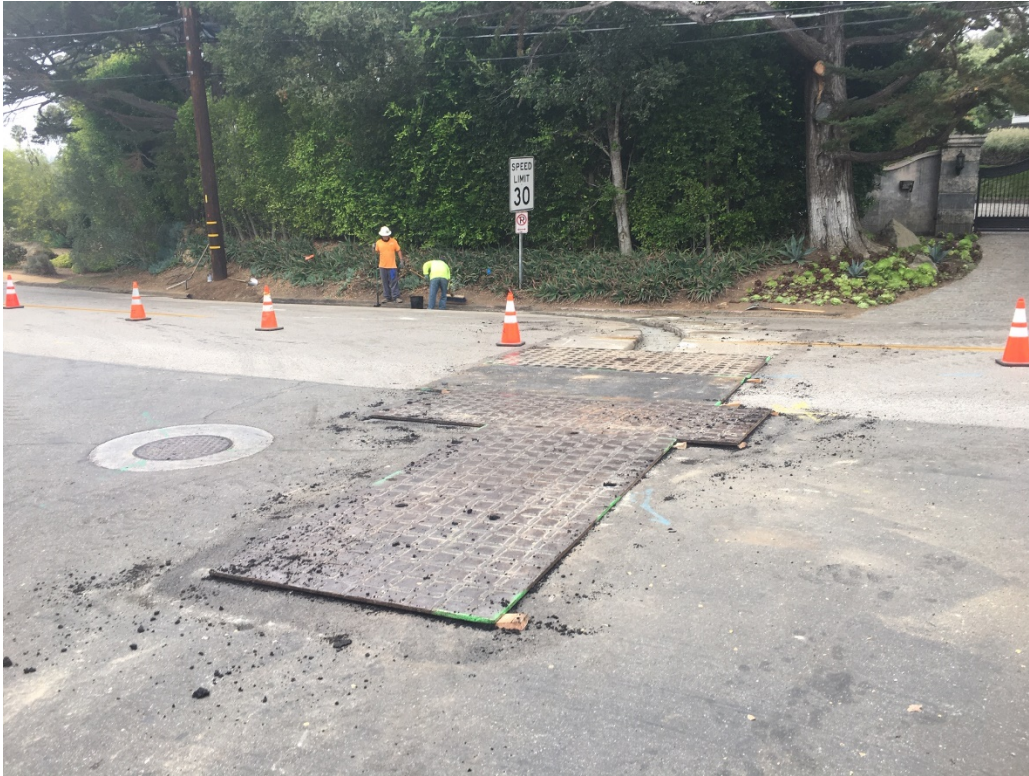
Observed installation of Southern California Edison underground electrical conduit near the South Coast Conduit in the San Ysidro Road and Bolero Road area in Montecito
