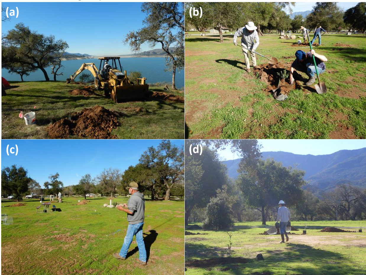
Exhibit 1: Lake Cachuma Oak Tree Restoration Program Year 10 planting showing (a) COMB backhoe digging holes, (b) backfilling a newly planted tree, (c) County Park employee checking for underground utilities, and (d) distributing new trees to be planted.
