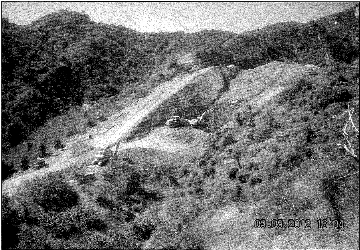
Photograph shows the pipe alignment, existing slope and the necessity of constructing a fill slope.
