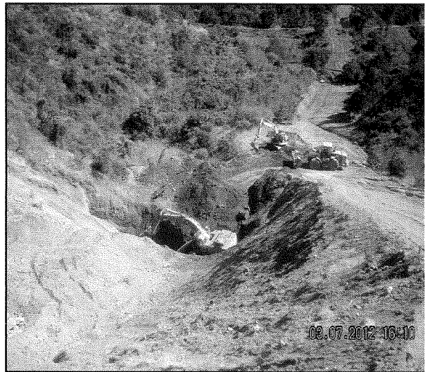
Beginning to fill keyway by mixing soil, rock and water and compacting.
