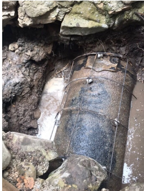
Conduit excavated by hand and reinforcement added prior to pouring concrete cap
