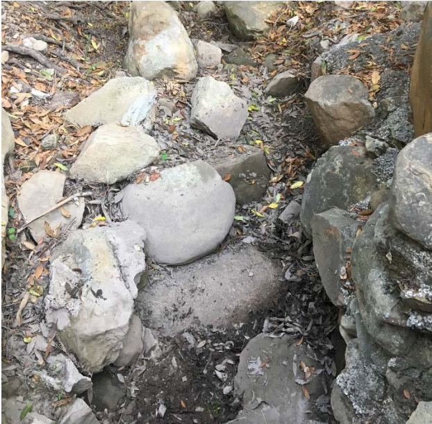
Exposed section of South Coast Conduit downstream of culvert outlet
