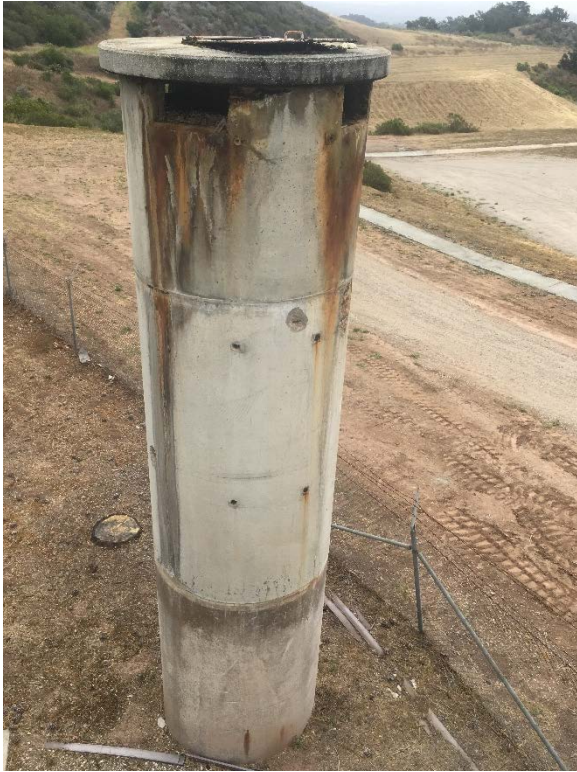
Open air vent on upper reach (raw water) with corroded vents/lid
