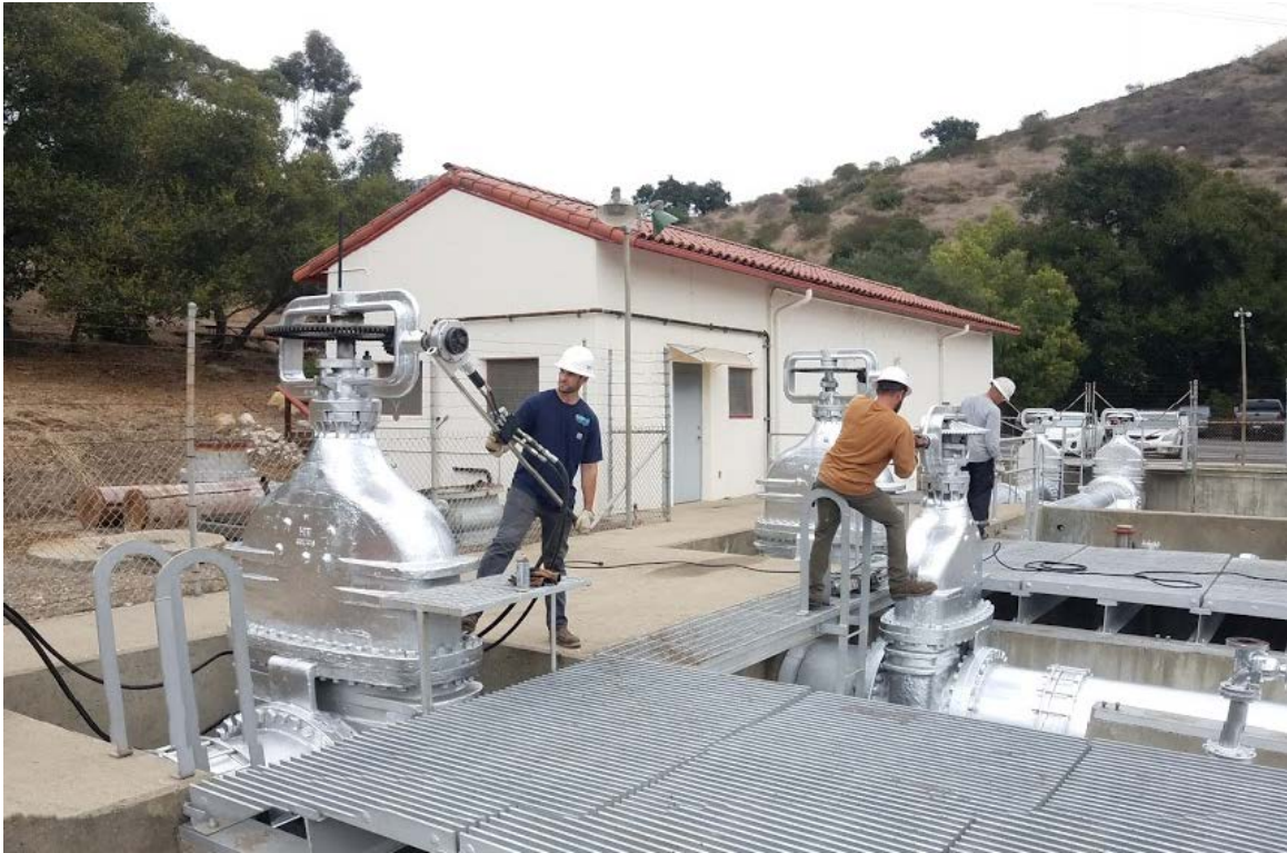
Exercising valves at Lauro Control Station
