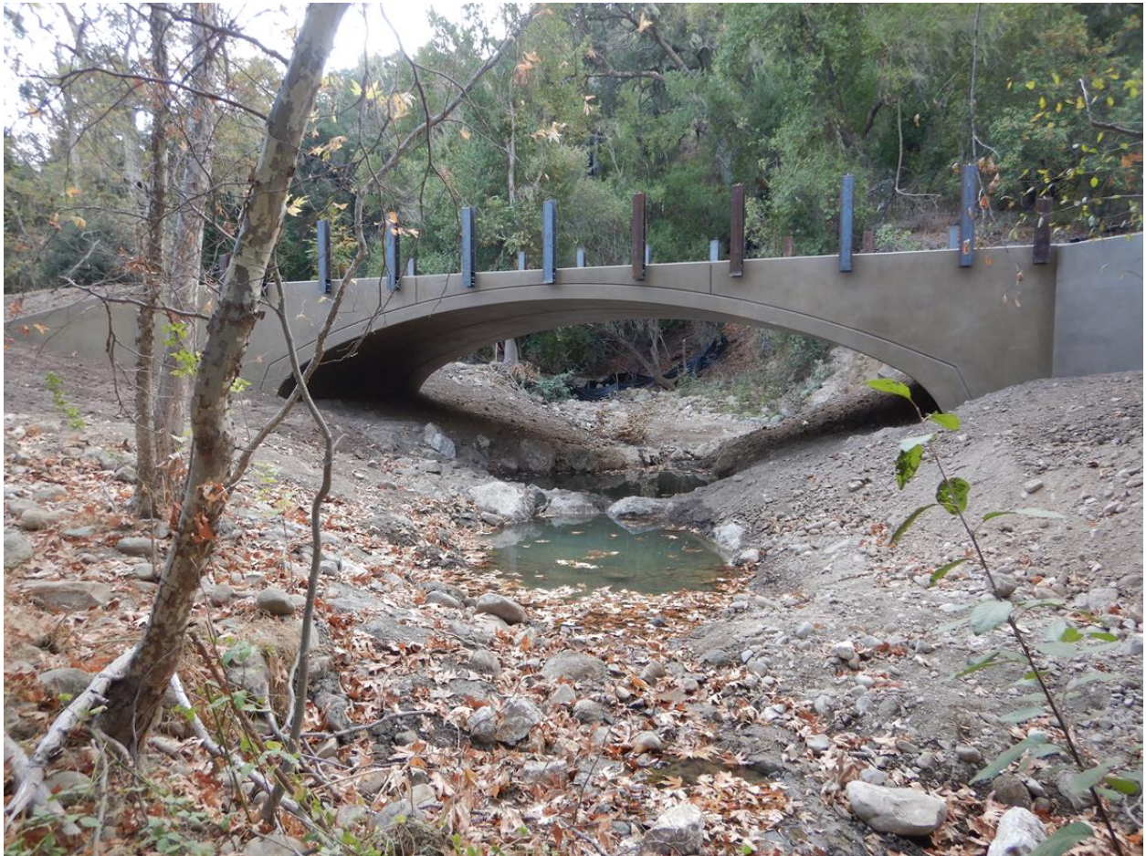
Figure 10: Current stream condition showing concrete staining and graffiti proofing, and installed bridge rail posts.
