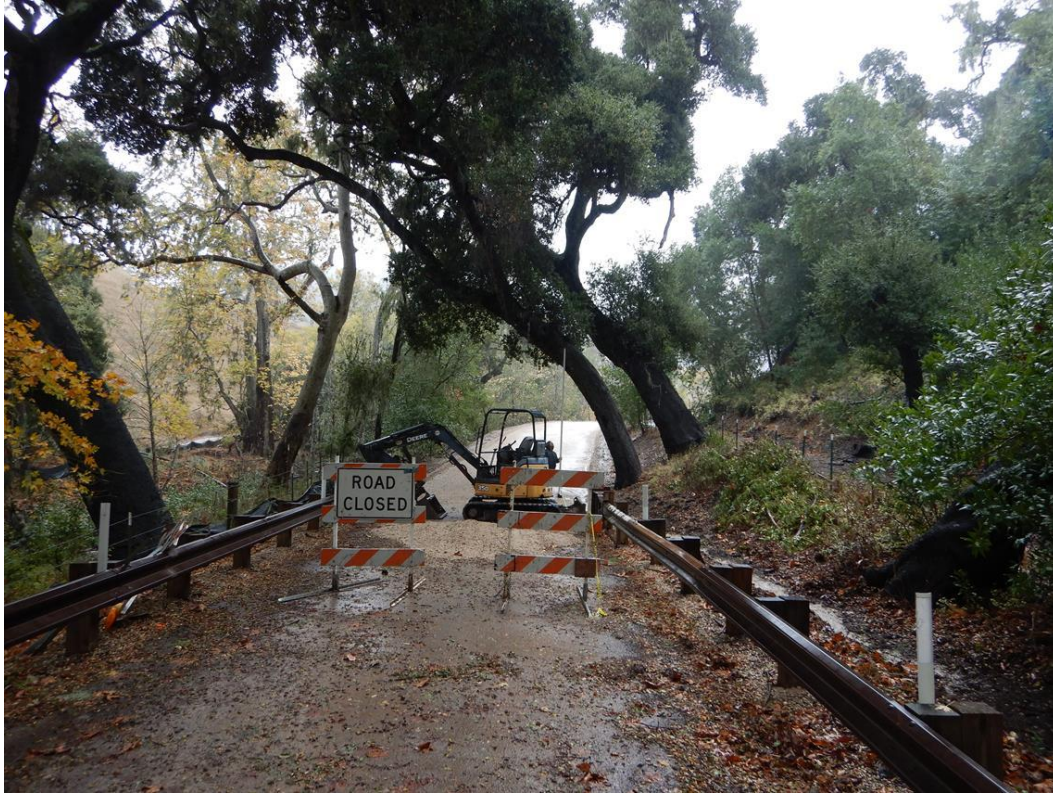
Figure 6: County required modifications for the tie-in to the Crossing 7 Project; move guardrail, remove tree, and additional asphalt.
