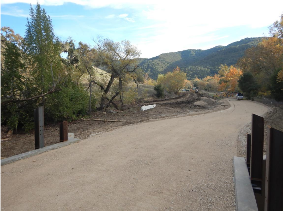
Figure 9: Drainage improvements for erosion control on the south side of the project.
