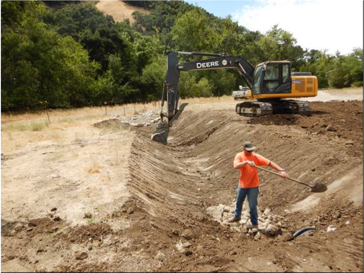
Figure 5: Excavating the Ranch Road drain settling basin and installing inlet and outlet native cobbles.
