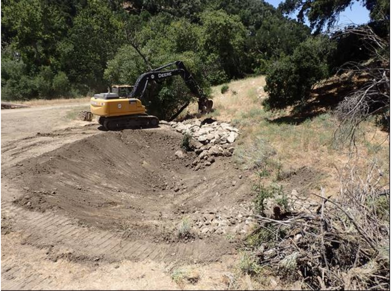
Figure 3: Placing the inlet and outlet native cobbles of the no name tributary settling basin.
