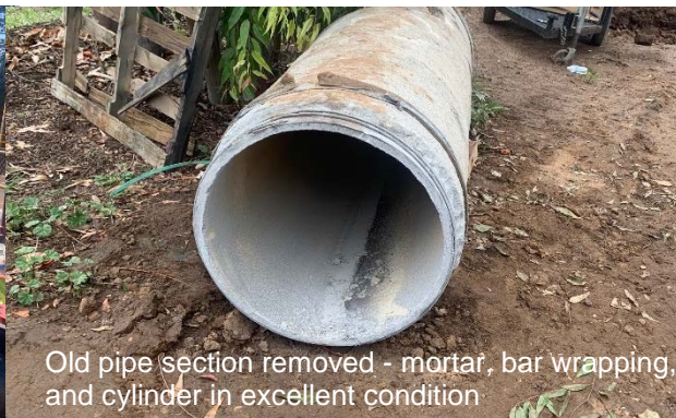
Old pipe section removed between line stops with water delivered through bypass
