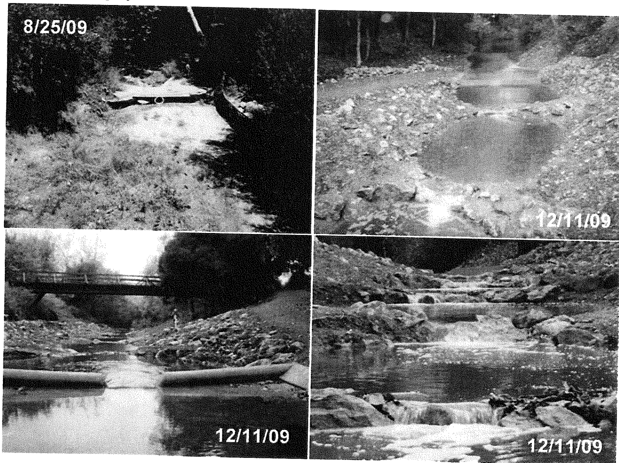
Figure 1: Projects photos from before the project started and after the completion of the project during the December 11, 2009 storm. Fish passage for juvenile and adult southern steelhead is now possible at all flows.
