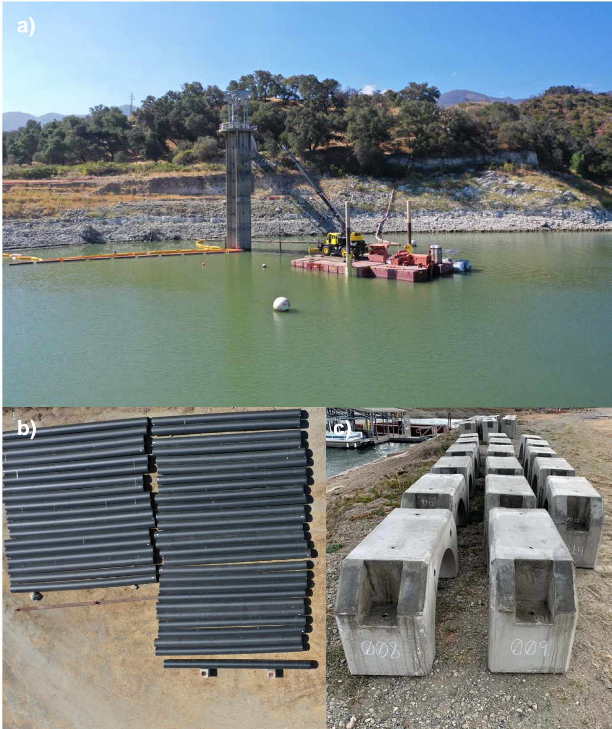
Figure 2: a) work barge dredging around the intake tower (J.Waller); b) HDPE pipeline stored at boat ramp staging area (J. Waller); c) concrete anchor weights delivered to site.
