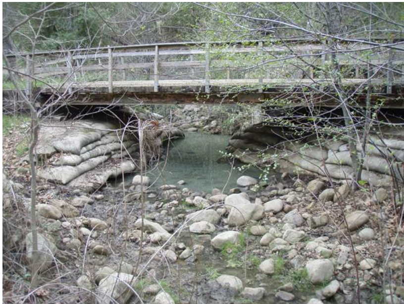
Figure 1: Temporary County bridge on South Refugio Road at Quiota Creek Crossing No. 8 looking upstream.
