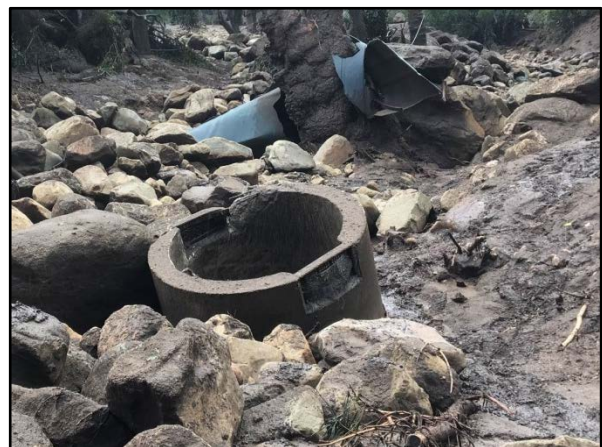
Damage to SCC vault during 1/9/18 debris flows
