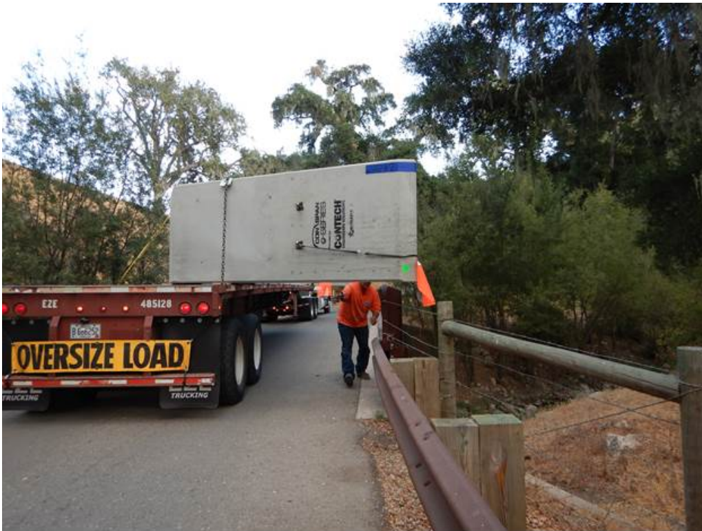
Figure 4: Bridge transport up S. Refugio Road over the Quiota Creek Crossing 2 bridge.
