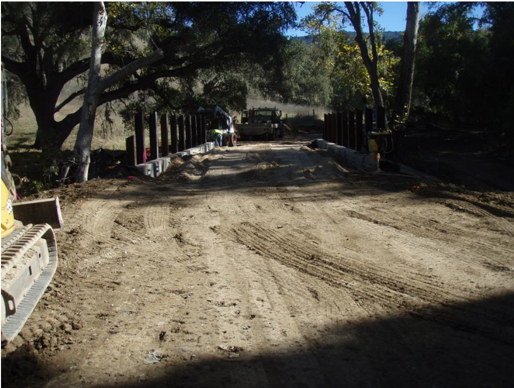
Figure 3: Final back filling of the arched bridge and installing the bridge rail posts.
