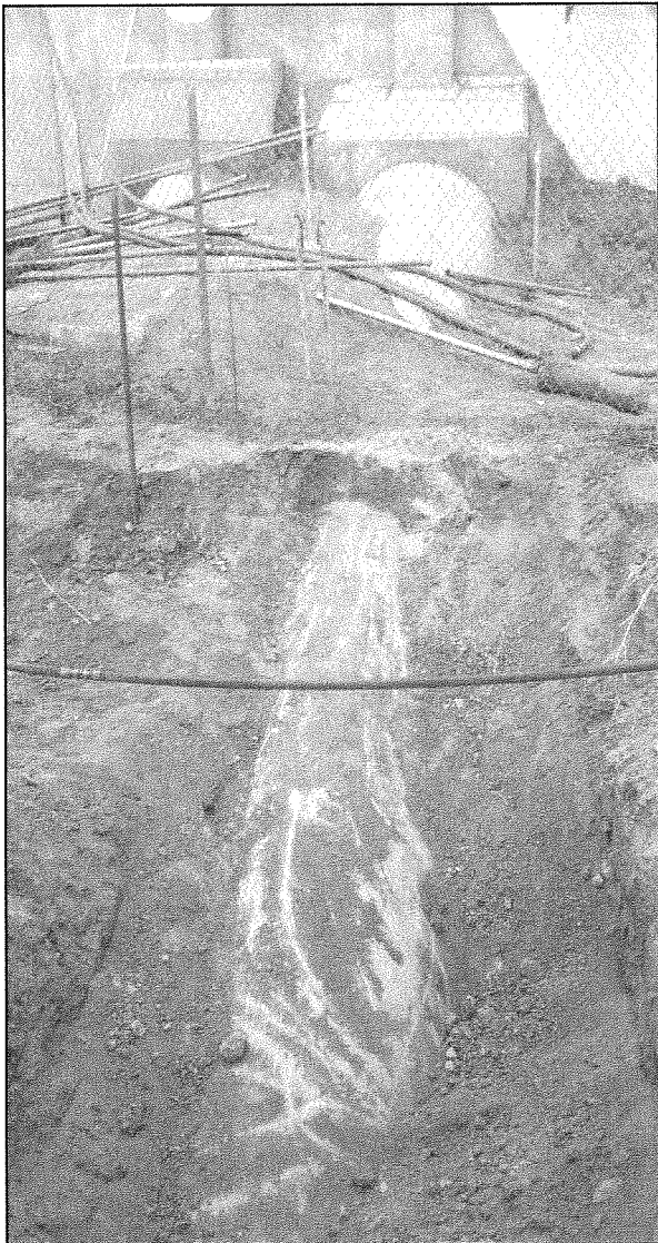
South Coast Conduit Exposed
