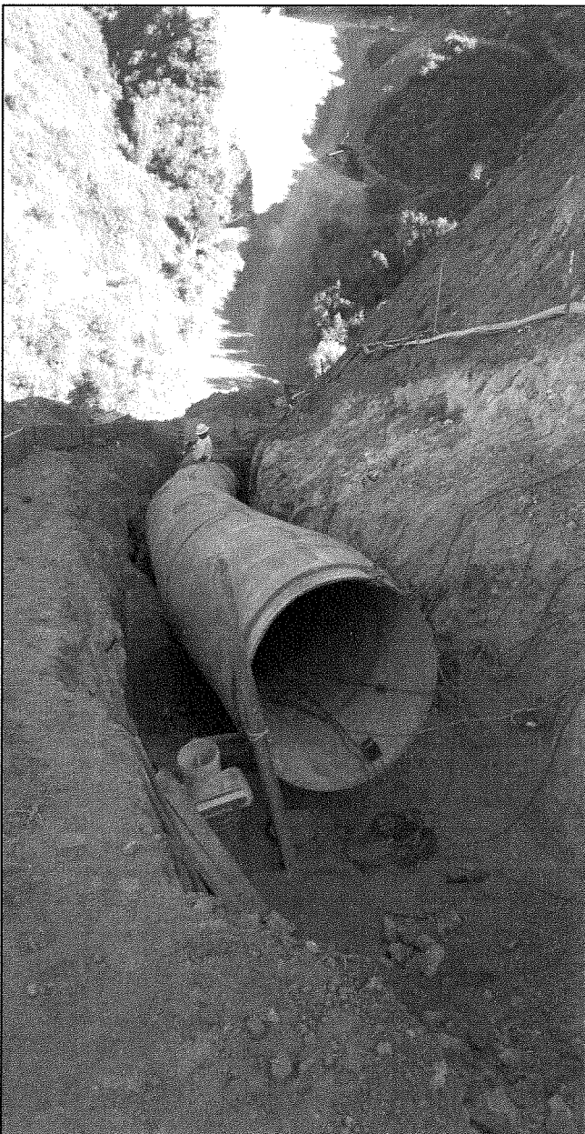
Last sections of underground pipe before above ground pipe at the Glen Annie Turnout
