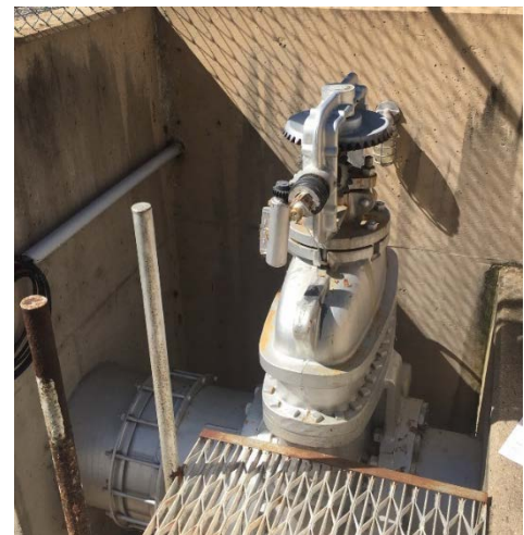
Ortega Control Station – Valve #1
