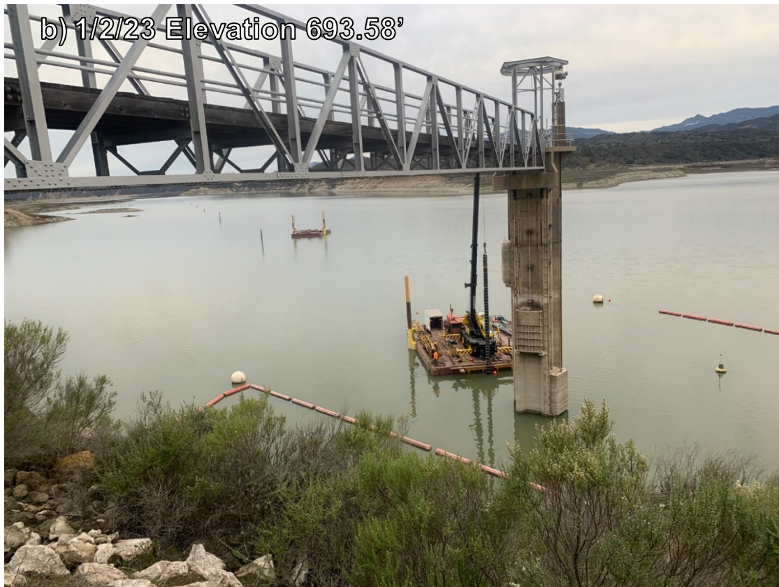
Figure 9: a) contractor setting up to drive piles at the intake tower on the 1/2/23 holiday with the lake at 693.58'; b) intake tower on 1/10/23 following 12.5" of rain at Cachuma Lake which resulted a 32.25' rise in a 24-hour period which exceeded the previous historical single day change by 10 feet.
