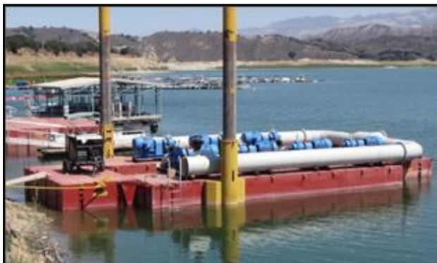
Emergency Pumping Facilities Barge
