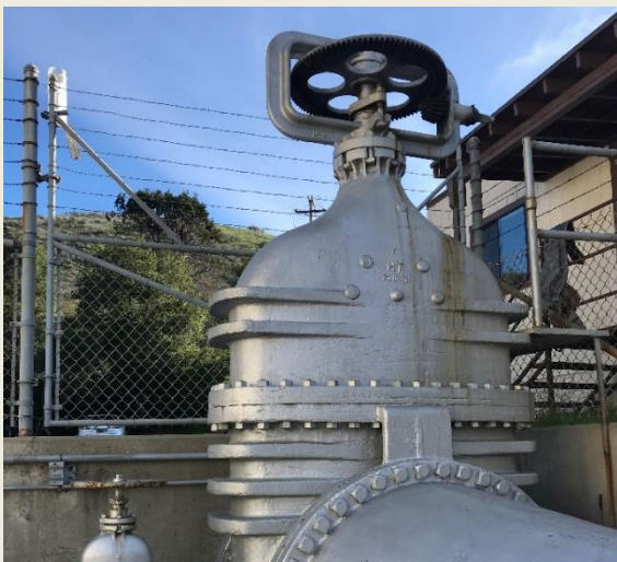
Figure 4. Lauro Control Station Gate Valve
