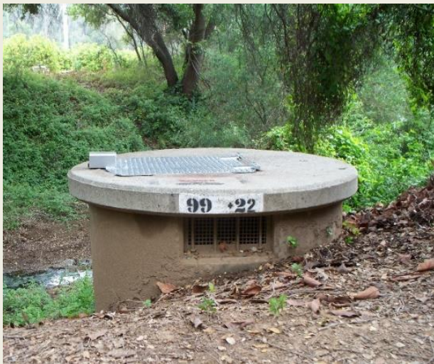
Figure 7. Blow Off Structure at Station 99+22
