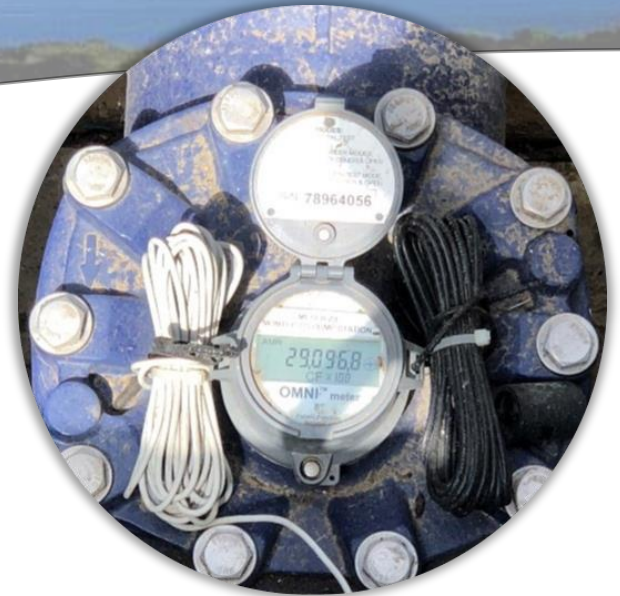
Figure A.11 Montecito Pump Station Meter
