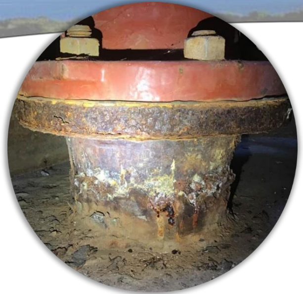
Figure A.10 Corroded Blow Off Riser Nozzle at SCC Upper Reach Station 639+50 Before Repairs
