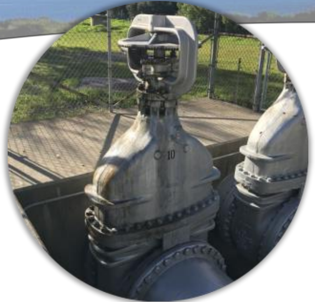
Figure A.12 Lauro Control Station Gate Valve
