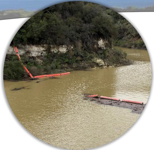
Figure A.16 Log Boom Shackle Failure
