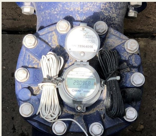
Figure 6. Montecito Pump Station Meter
