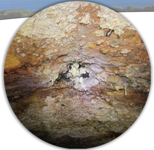
Figure A.14 Clogged Weep hole in Tecolote Tunnel
