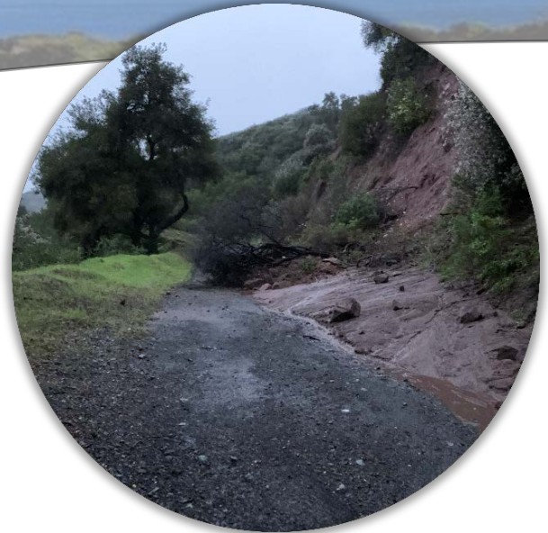
Figure A.8 Glen Annie Road Damage following January 2023 Winter Storms
