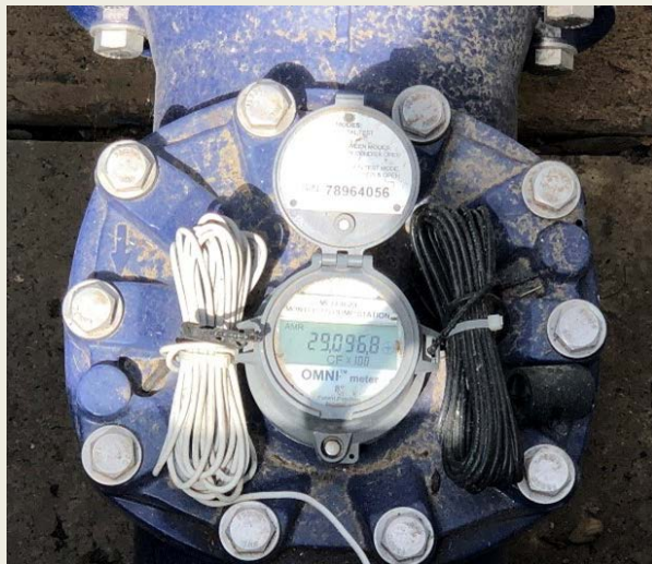
Figure 6. Montecito Pump Station Meter
