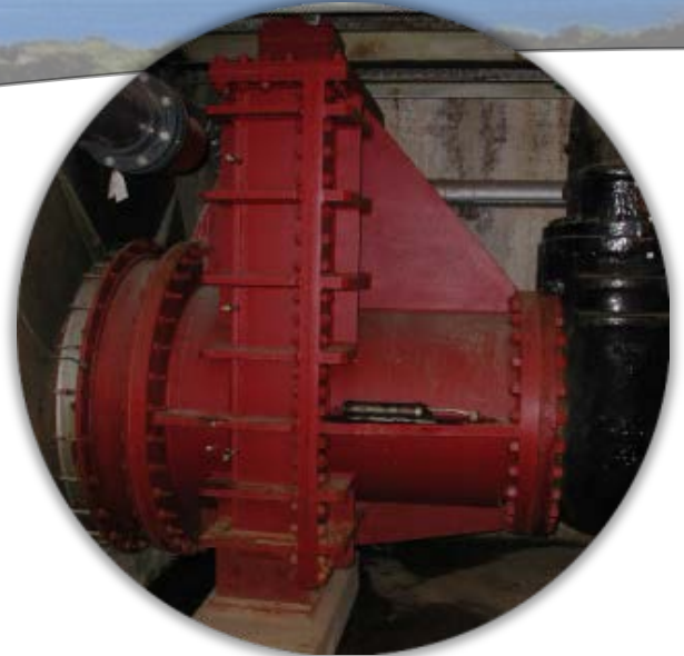
Figure A.17 North Portal Jet Flow Control Valve
