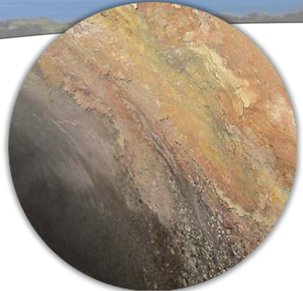
Figure A.15 Concrete Lining Deterioration within the Tecolote Tunnel
