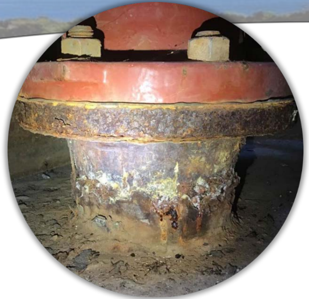
Figure A.10 Corroded Blow Off Riser Nozzle at SCC Upper Reach Station 639+50 Before Repairs
