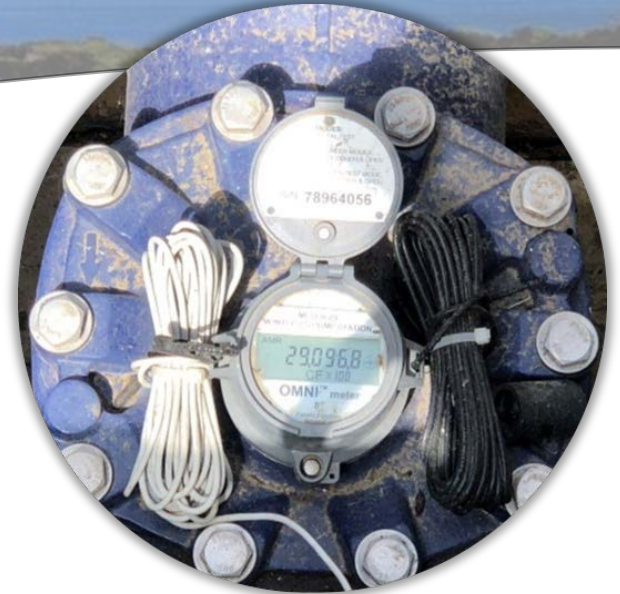
Figure A.11 Montecito Pump Station Meter
