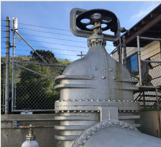
Figure 4. Lauro Control Station Gate Valve
