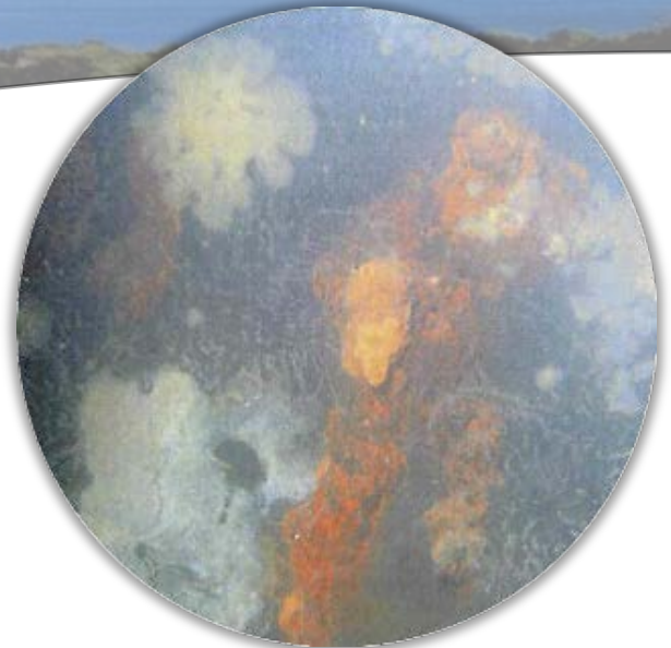
Figure A.9 Corroded Steel Bearing Plate on Lauro Reservoir Intake Structure
