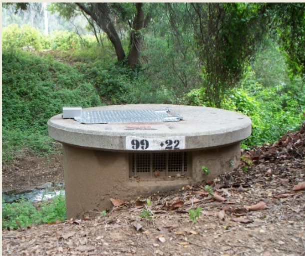
Figure 7. Blow Off Structure at Station 99+22
