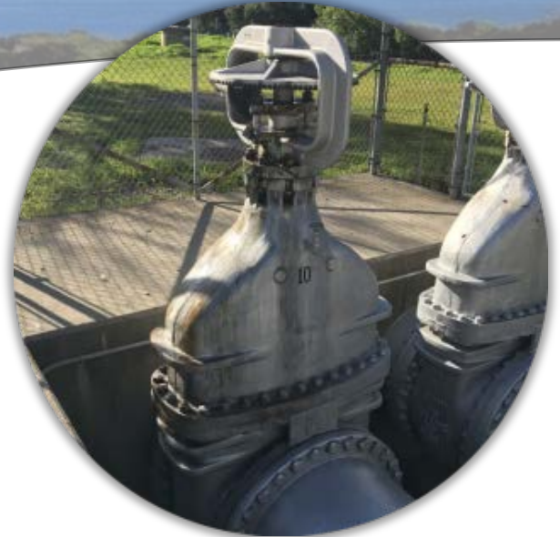
Figure A.12 Lauro Control Station Gate Valve
