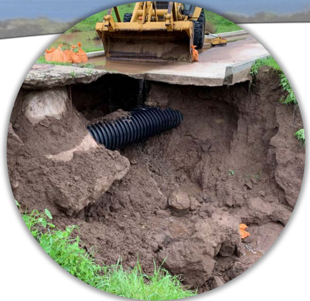
Figure A.5 Lauro Reservoir Bypass Channel Washout January 2023 Winter Storms
