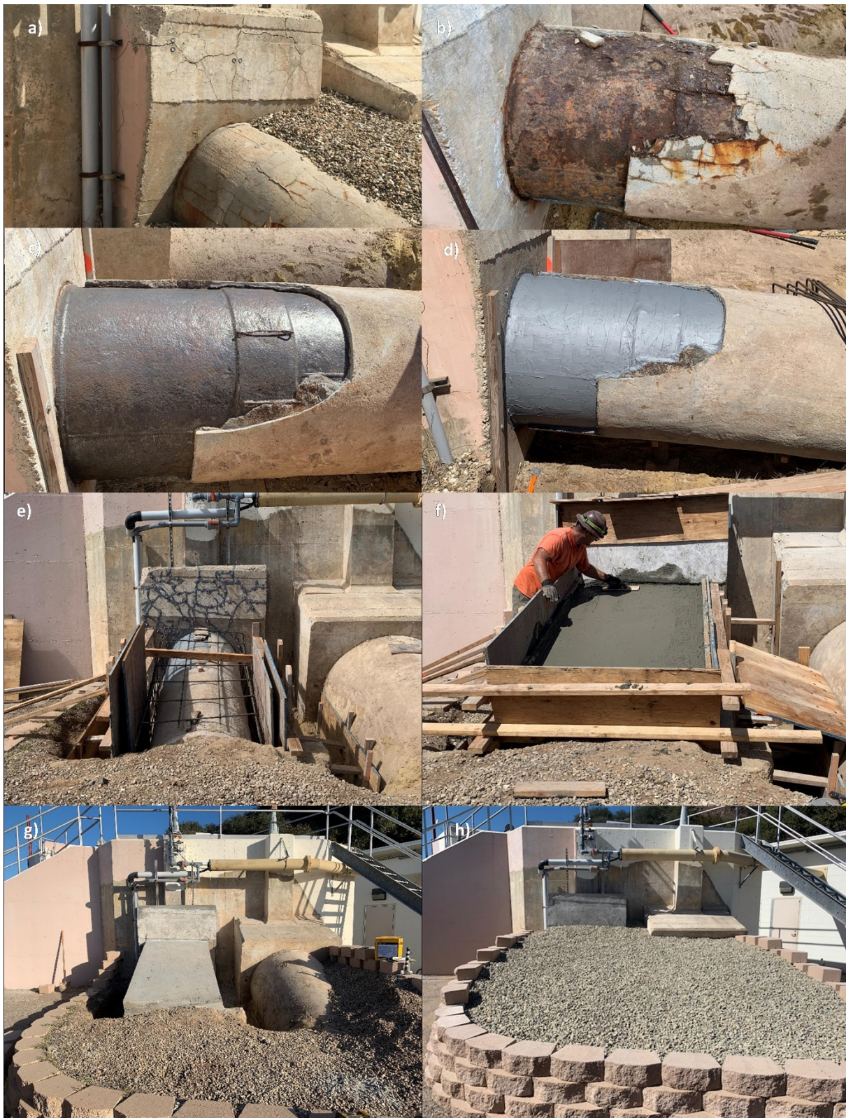
Figure 2. Goleta West Conduit Repair at GATO – a) cracks in concrete and mortar coating showing signs of corrosion; b) damaged mortar removed showing rust corrosion of pipeline under mortar; c) pipeline cleaned to bare metal; d) pipeline coated with metal alloy epoxy resin (Belzona 1111); e) cracks in concrete injected with structural epoxy resin; f) concrete encased from turnout box to buried thrust block; g) concrete forms removed; h) gravity block wall raised and gravel fill add to cover concrete and adjacent South Coast Conduit.
