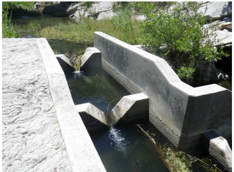
Figure 5: Salsipuedes Creek fish ladder at Jalama Road showing weirs that need to be fixed.
