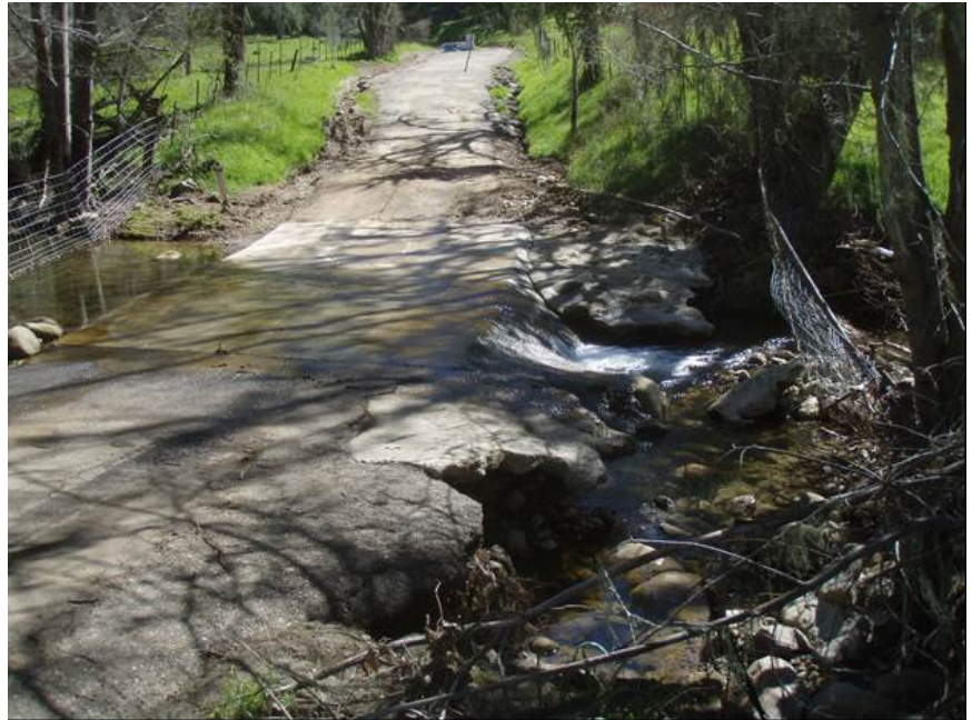
Figure 3: Quiota Creek on Refugio Road showing side-view of Crossing 9.
