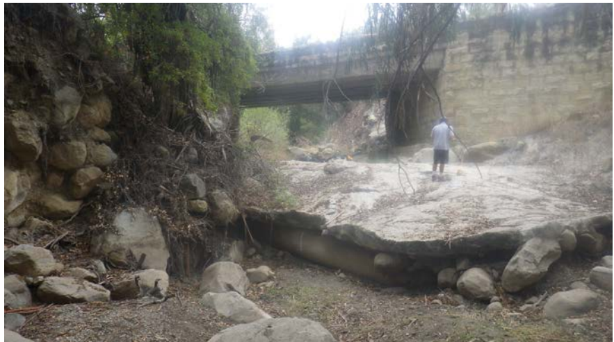
Figure 6: Mission Creek at Highway 192 showing the fish passage impediment, SCC and protective concrete on top.
