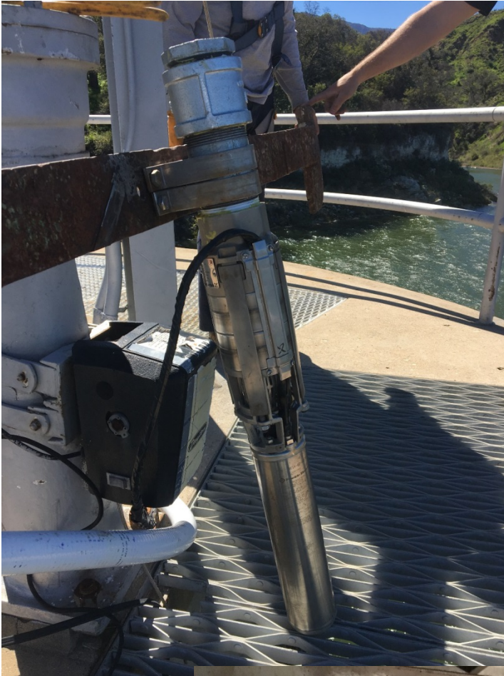
New wash water pump – Intake Tower
